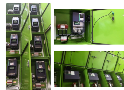
customized solar pump control panel
